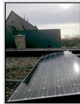
Solar panels installed in St. Luke's Church in Dixon, Ill.
